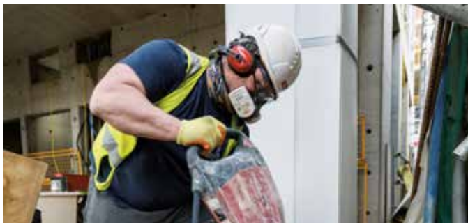
The health, safety and wellbeing of our contractors is paramount – The Featherstone Building EC1
