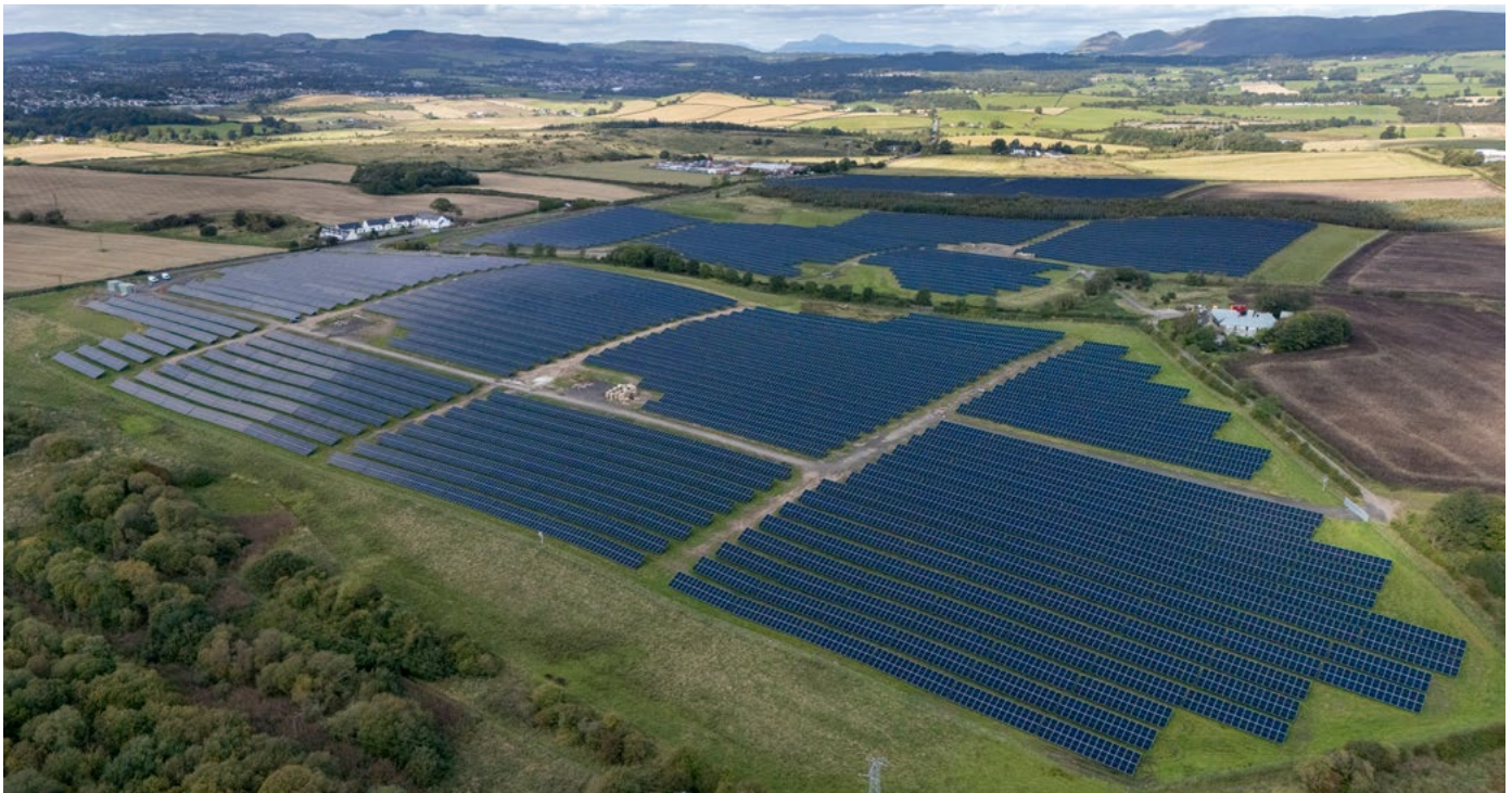
Lochfauld Solar Park
